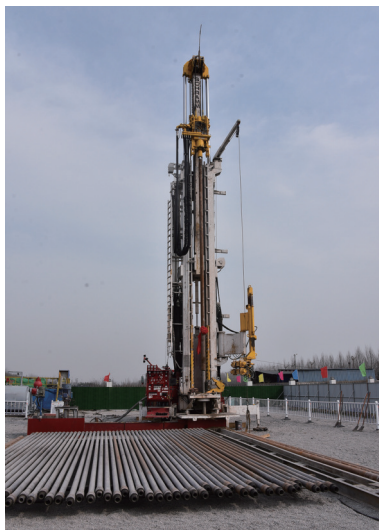
图 6 大直径救生孔施工现场 Fig.6 On-site construction of a large-diameter lifesaving hole
